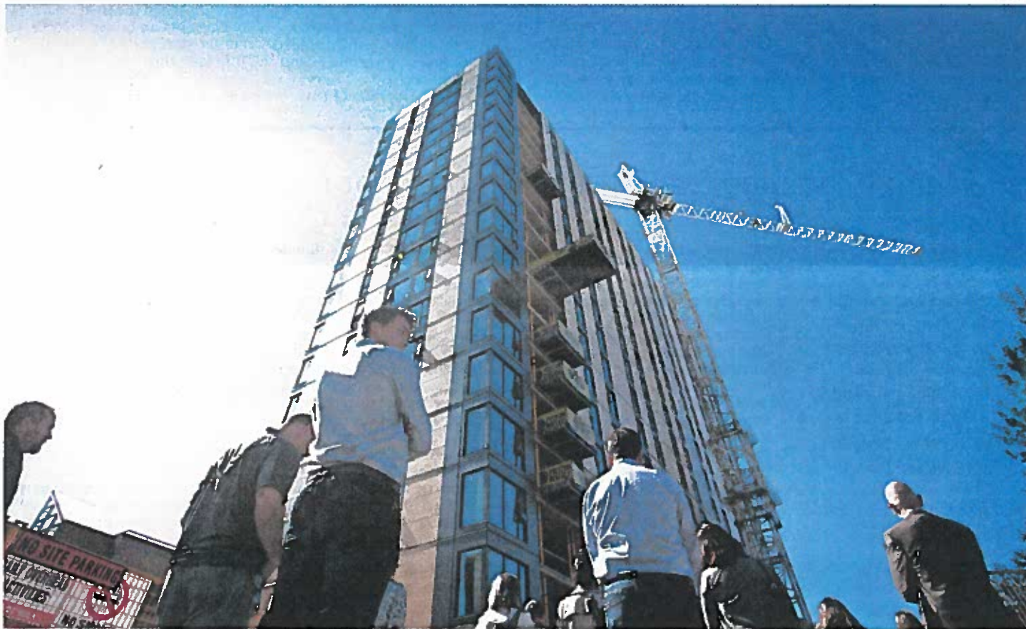
People stand outside the Brock Commons student residence building, which is under construction, at the University of British Columbia during a ceremony to mark the completion of the wood structure on Thursday. It is the first mass wood, steel and concrete hybrid project to extend taller than 14 storeys in the world. The 18-storey building is scheduled to welcome more than 400 students in September, 2017. DARRYL DYCK FOR THE GLOBE AND MAIL
